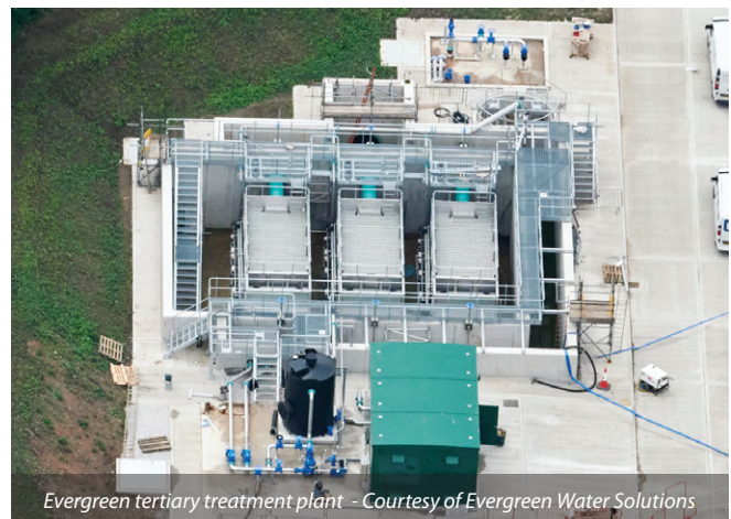
External mounted backwash pumps Courtesy of Evergreen Water Solutions
