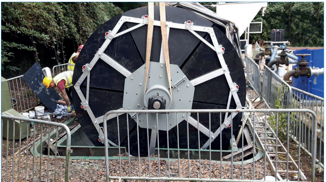
Anglian Water, Brinkley
