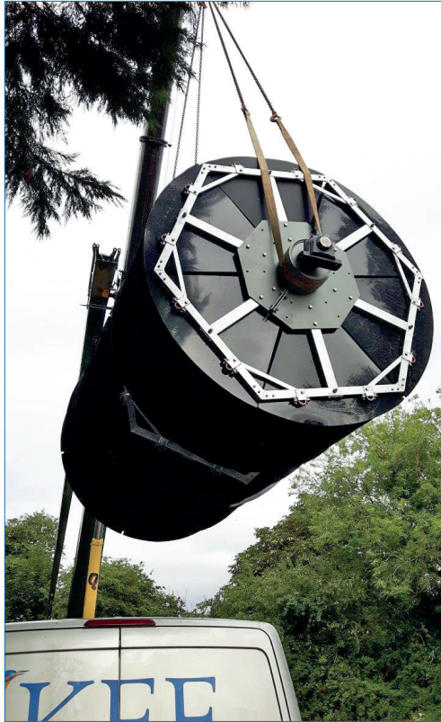
Anglian Water, Brinkley
