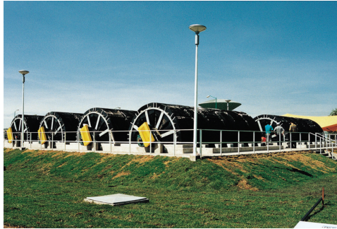
Large RBCs for biological treatment.
