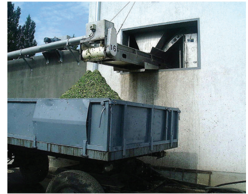
Vegetable processing wastewater screening prior to being treated in a multi-stage Submerged Aerated Filter Plant.
