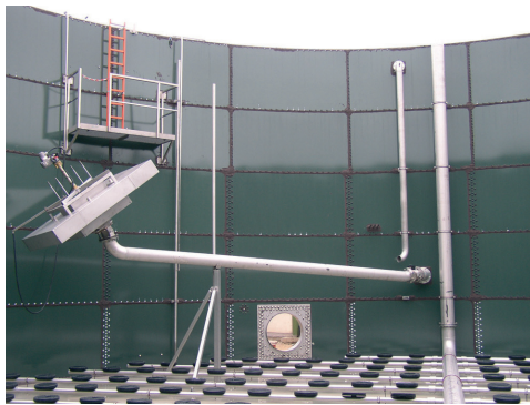
The decanter and access manway of a fruit juice wastewater treatment SBR Plant.
