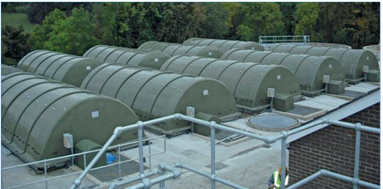
10 KEE RBCs at the new Keady Wastewater Treatment Works.
